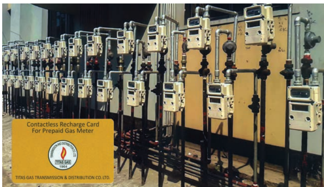
Prepaid gas meter and card of TGTDC
