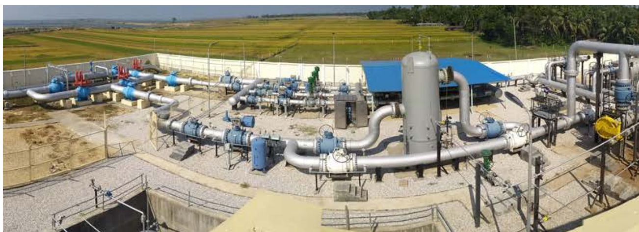
Moheshkhali CTMS, Cox's Bazar of GTCL
