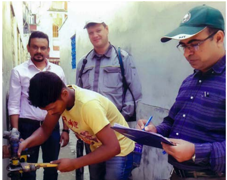
Gas Leakage detection, measurement and repair work under CDM project of TGTDCCL
