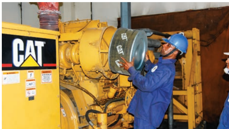
Maintenance of LPG plant of RPGCL
