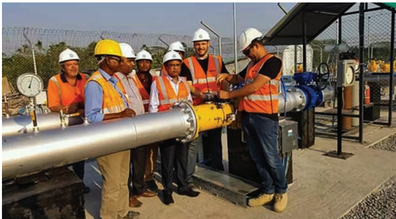
Commissioning Works of Aggreko 95MW RPP RMS, Borhanuddin, Bhola under SGCL
